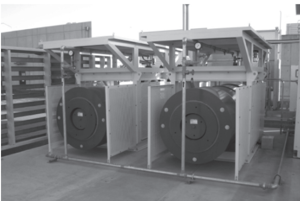
Fig.6 0.45 m 3 hydrogen pressure vessels
