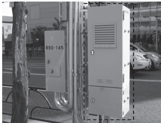
Fig.23 Fuel cell backup power for traffic signals
