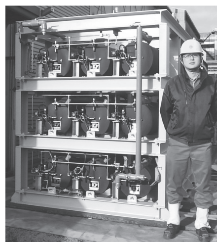
Fig.17 MH tank system with a storage capacity of 100 kg of hydrogen
