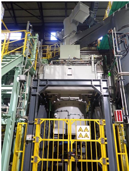
Current melting and casting facility at MCA
