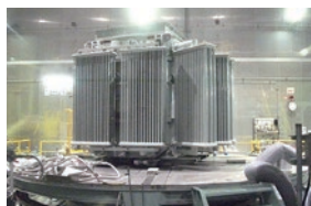
High-voltage transformers (at initial facility)
