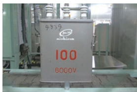
High-voltage capacitors (at initial facility)
