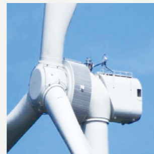
J82-2.0D wind turbines system
