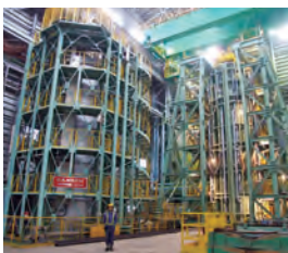
熱処理炉 Heat Treatment Furnace
