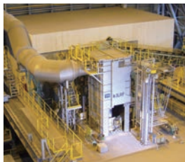
取鍋精錬炉 Ladle Refining Furnace
