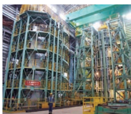
熱処理炉 Heat Treatment Furnace
